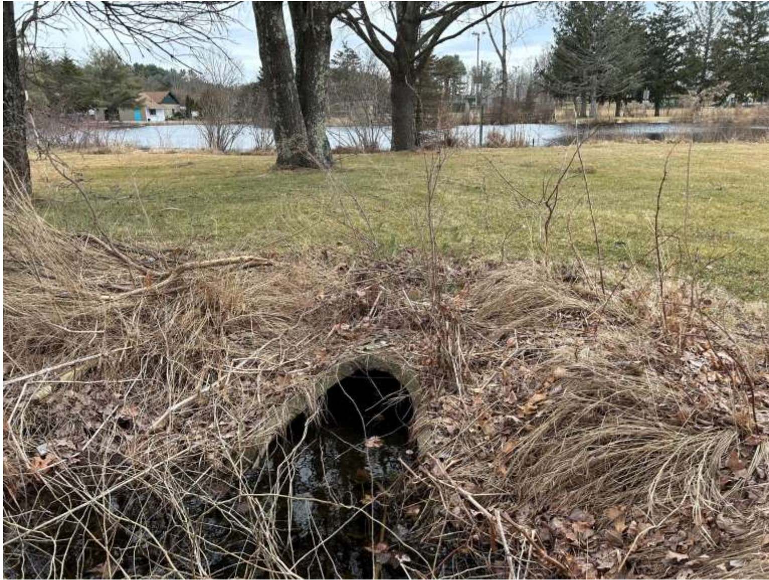
12. Standing in Drainage Swale North of Pond, Looking South. 24" Flared End Section From Swale to Pond Inlet
