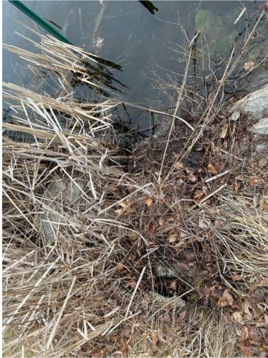
11. Inlet to Pond. Spigot End of 24" RCP (Submerged & Broken)
