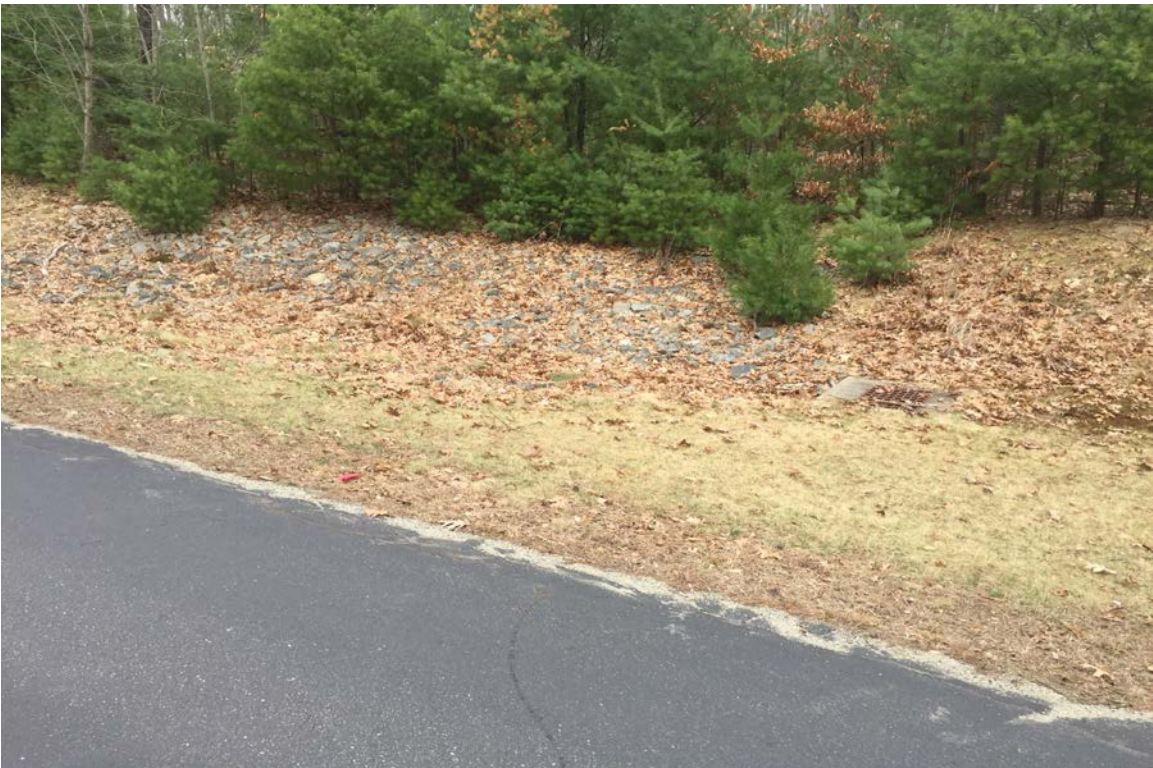
Photo 4: View of Wetland 2 crossing from high school access road looking northeast; note rip rap armored cut slope and catch basin.
