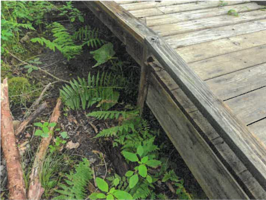
III. Material fill at bridge abutments
