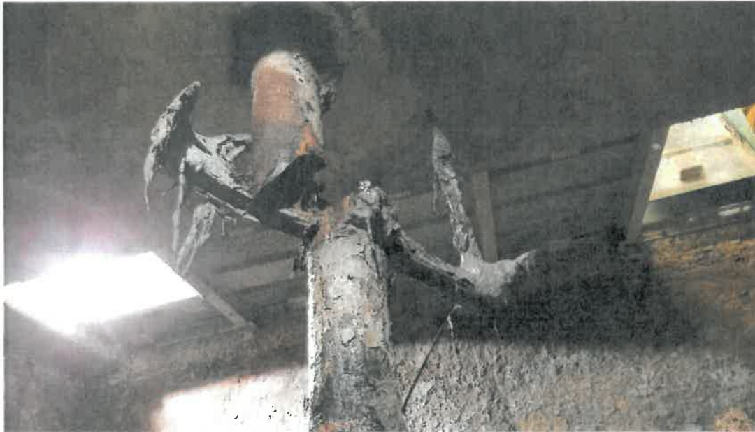
Picture – Broken Sludge Mixer
