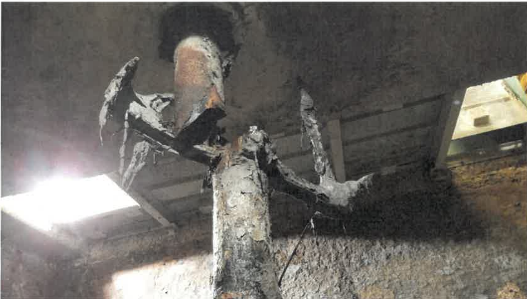
Picture – Broken Sludge Mixer
