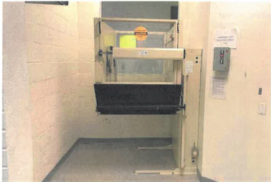
One of the school's two existing chair lifts providing access for the main entrance level to the intermediate floor level to the north. The lower level of the school's south wing is currently inaccessible from upper floors.
