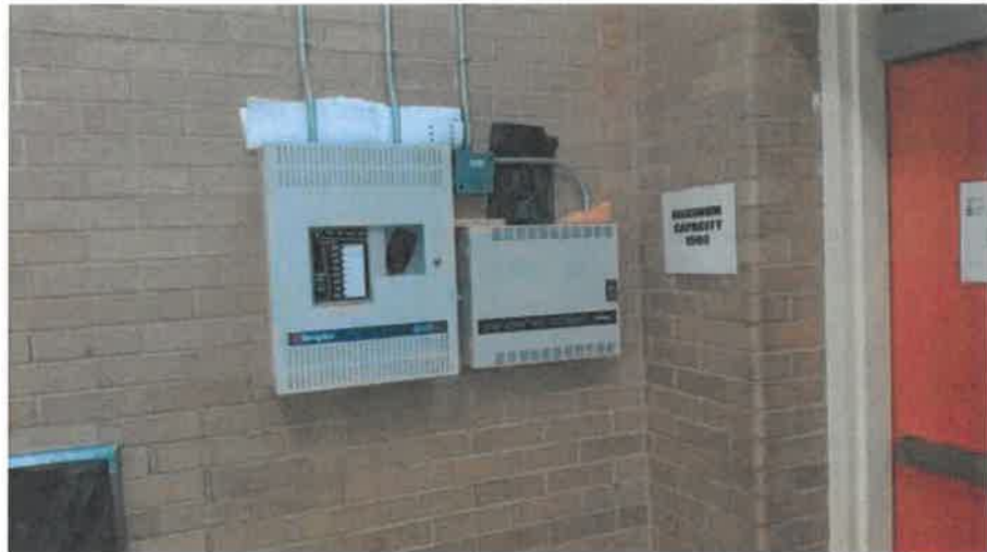
Existing fire alarm voice evacuation panel and NAC booster panel in gym.
