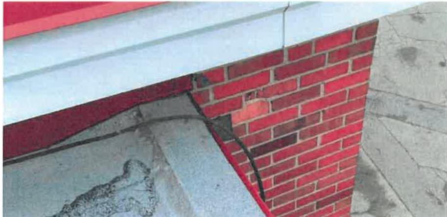
Minor cracking and a spalled face brick observed below the roof cornice of the middle wing's north elevation.
