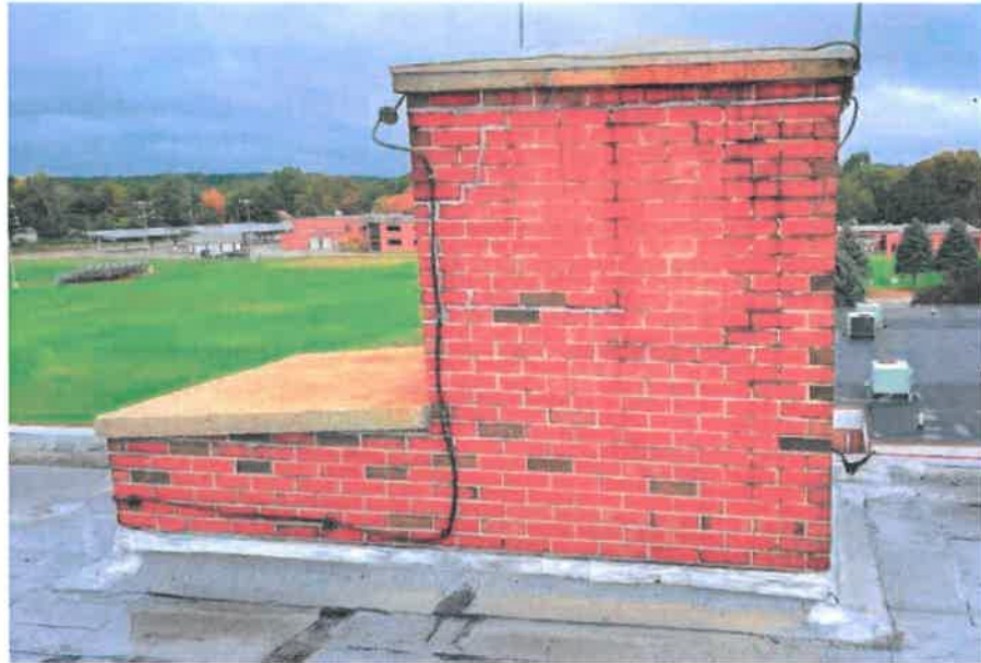
Evidence of staining and repair of separated mortar joints at a chimney above the Gymnasium – Auditorium roof.
