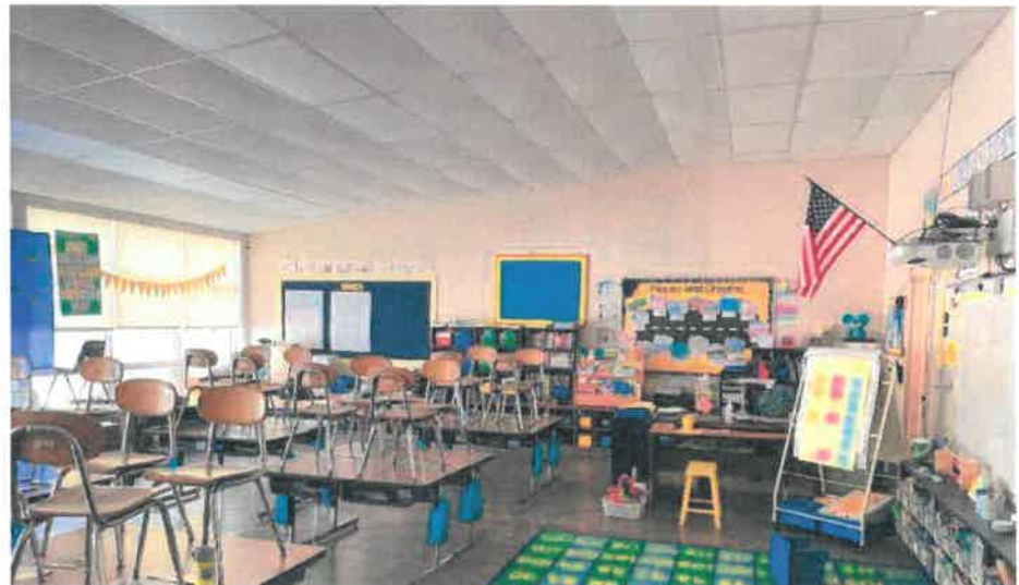
Classrooms 209 and 210 in the existing school have a unique, partially vaulted 24 by 48-inches suspended acoustic panel ceiling. The pads show signs of sagging.
