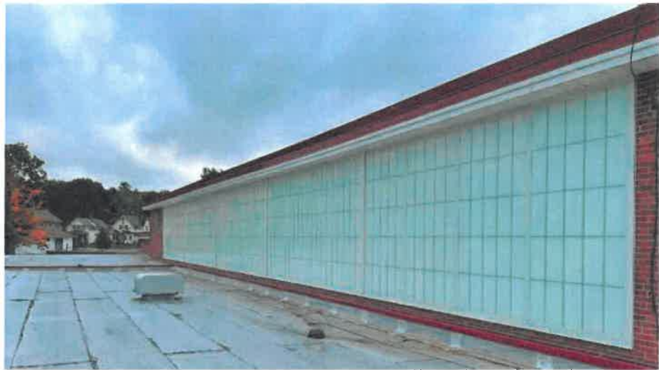
An exterior view of the translucent panel glazing system installed along the north wall of the Gymnasium – Auditorium.
