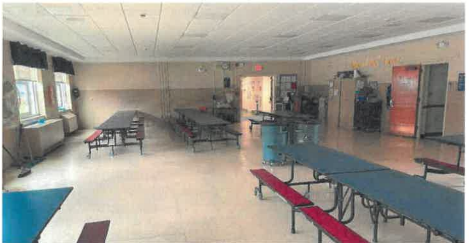
A contemporary 24 by 24-inches tegular acoustic ceiling with 24-inches perimeter gypsum board soffit assembly in the existing Cafeteria.
