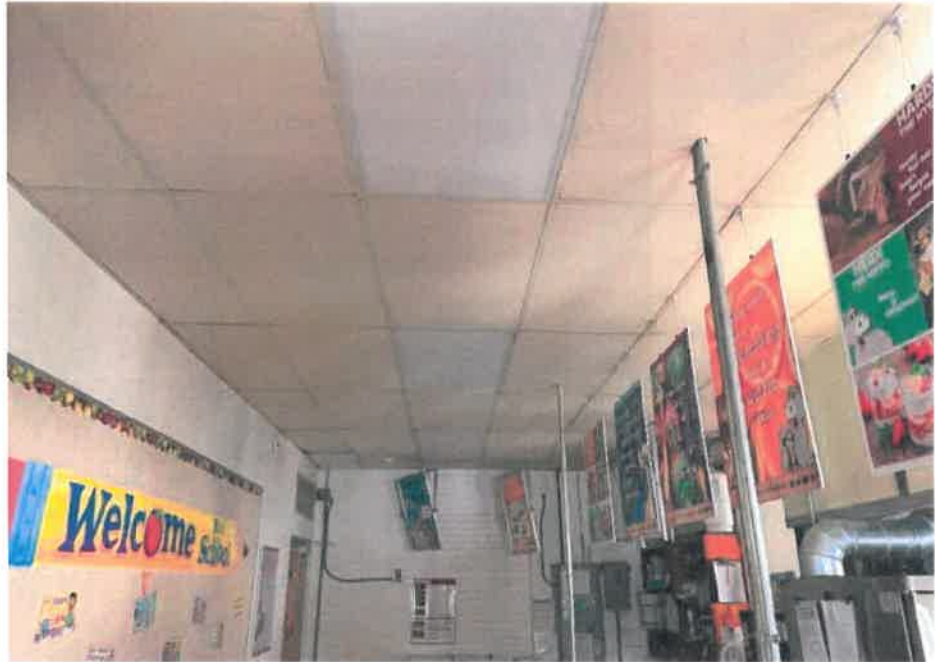
A 24 by 48-inches vinyl faced ceiling panels in a suspended grid is installed above the existing serving and kitchen of the school. The ceiling panels are heavily stained from cooking activities.
