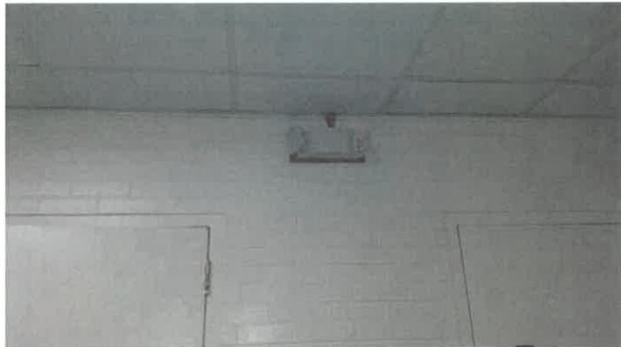
Dual head emergency lighting unit in corridor.
