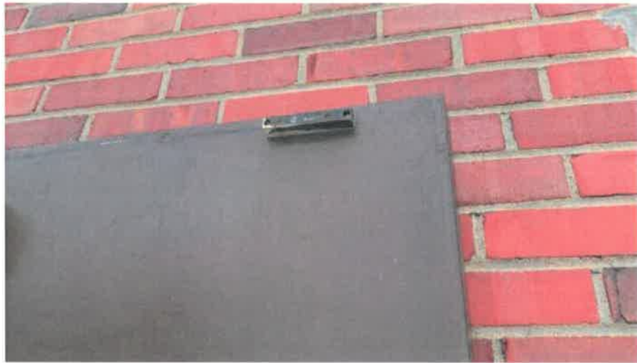
Existing door contact.
