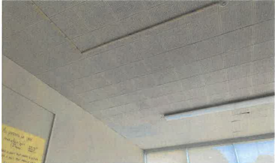
An example of an original classroom ceiling consisting of 12 by 12-inches adhered acoustic tiles.
