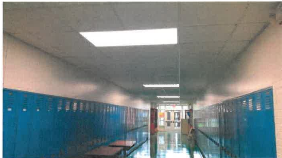
Existing recessed 2x4 LED luminaires in main level corridor.
