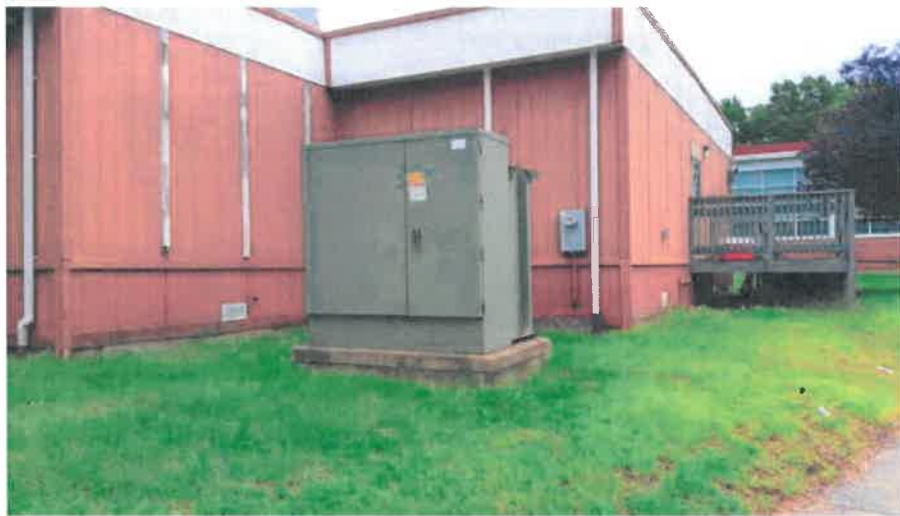
Existing West portable pad mounted transformer.
