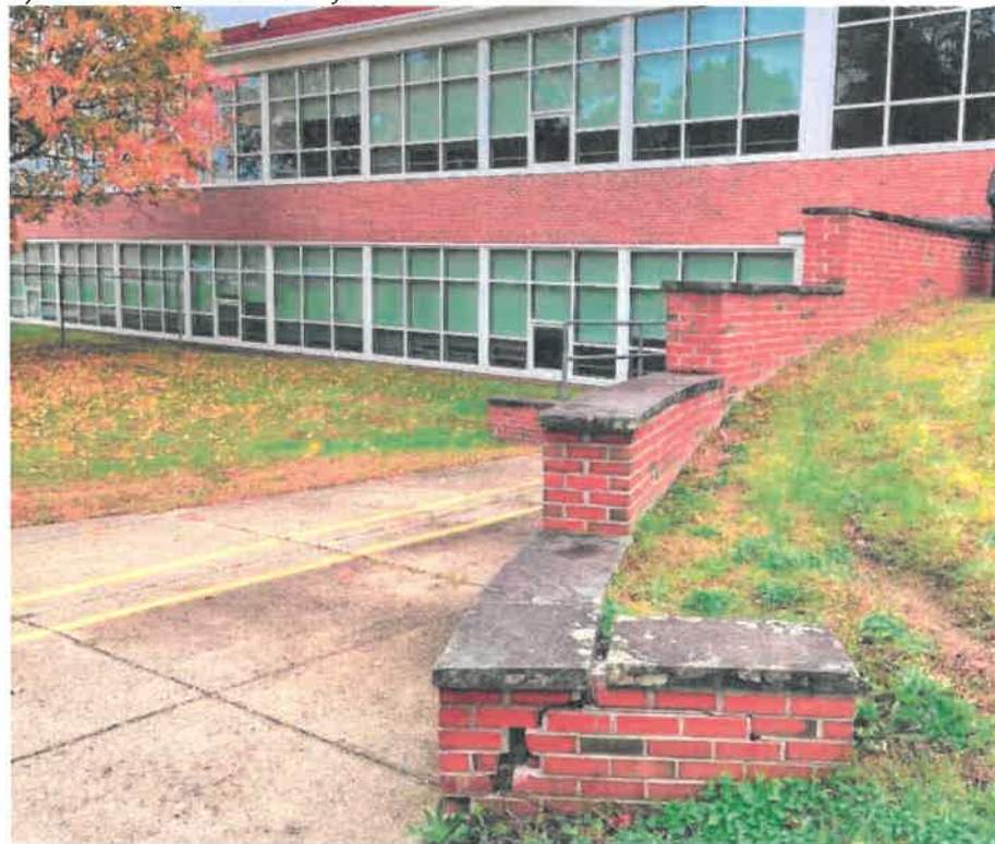
An exterior site wall with loose cap stones and cracking masonry.
