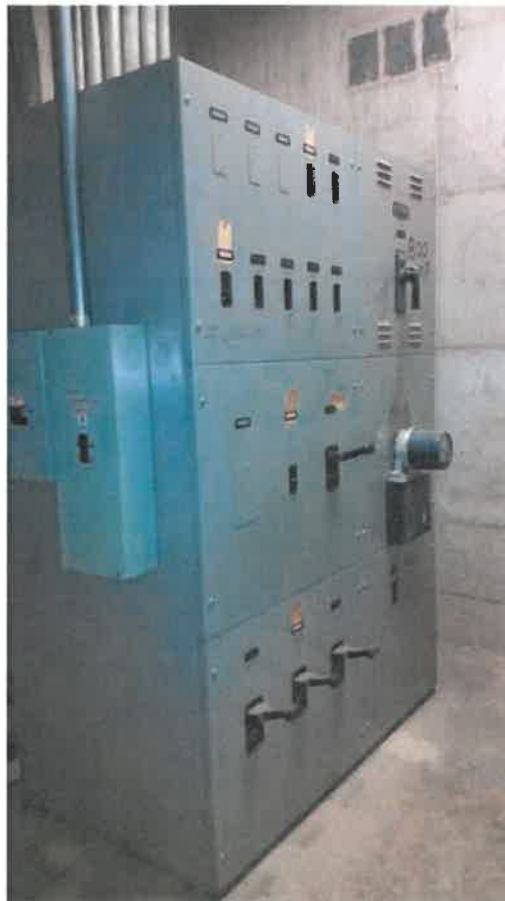
Existing 800A, 120/208V, 3Ph, 4W switchgear in main building.
