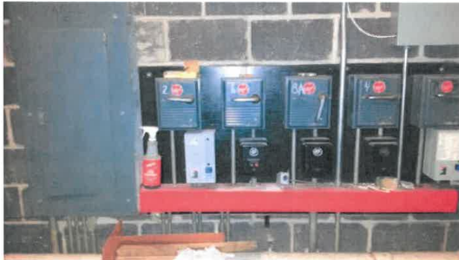
Existing disconnects and starters for HVAC equipment in upper level mechanical room.
