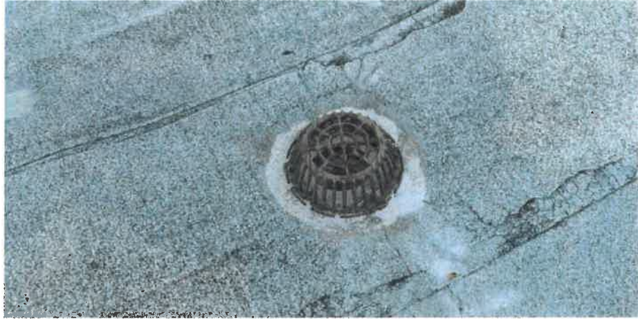
An example of a typical internal roof drain located within a depressed sump.
