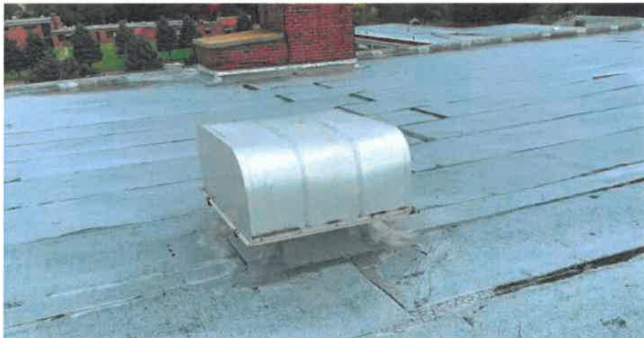
Roof vent for an existing exhaust within the modified bitumen roof system.
