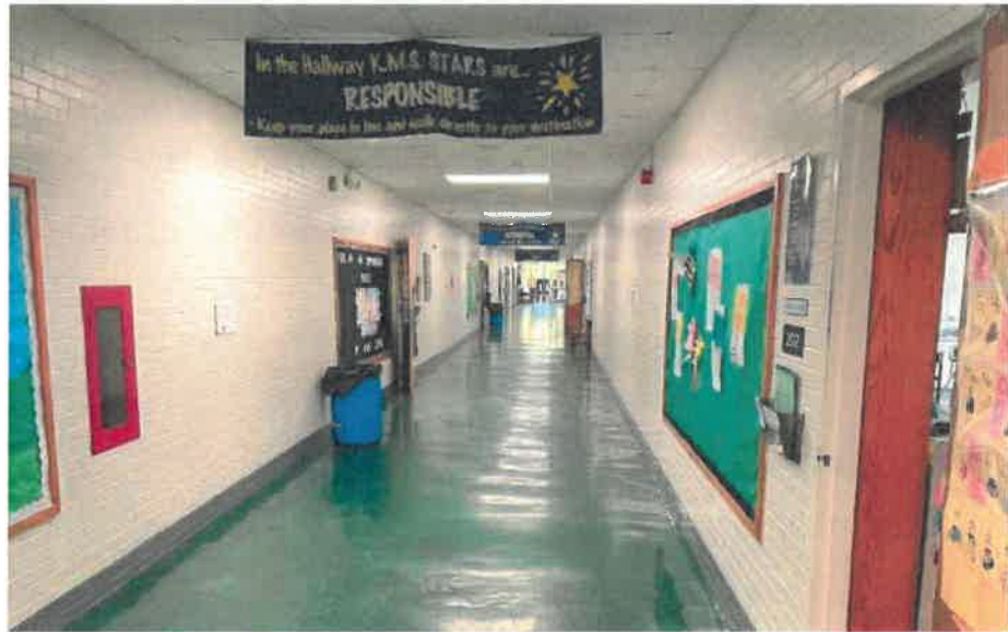
A representative double-loaded corridor serving academic spaces with existing resilient floor tile, painted brick masonry walls and suspended acoustic tile ceilings. Instead of a resilient base, the lower two courses of brick have been painted in a mid-tone gray color to distinguish it from the white wall surfaces.
