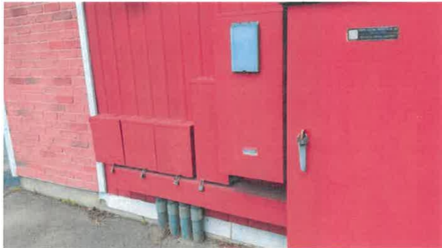
Existing East portable electrical service meter and disconnect enclosures.
